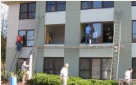
Even as the paint was being completed, the window crew arrived to begin installing the new windows.
