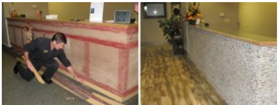
John Watterson, Plant Operations Director, preps the reception desk for new stone work. The new stone contrasts nicely with the new pine flooring.
